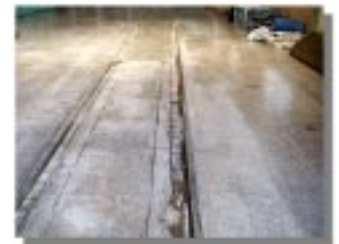
Broken concrete flooring along rails allowed water to migrate to a generator room.
