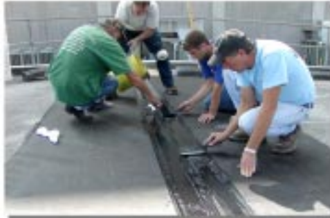
Lesco crew members go to work on the sealant joints at MUSC in Charleston.
