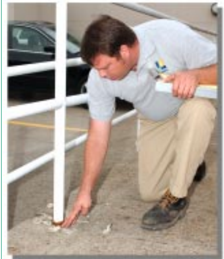
Concrete around this railing has crumbled, making the railing less secure and opening the way for water to penetrate and do more damage.
