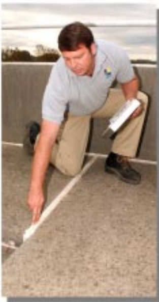
Sealant joints that are properly maintained prevent water from penetrating and creating problems below.
